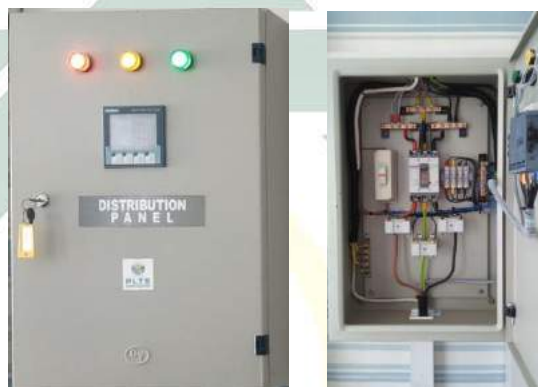
Picture 4.6 Distribution Panel
